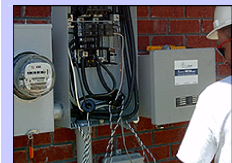
Alabama Electric Co-op technician installs a meter to monitor a tankless water heater.
